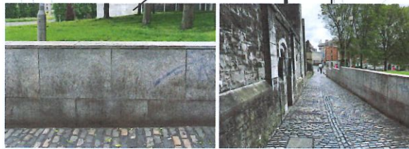
Retaining walls enclose John's Lane and do not allow a visual or physical connection with the existing open space
